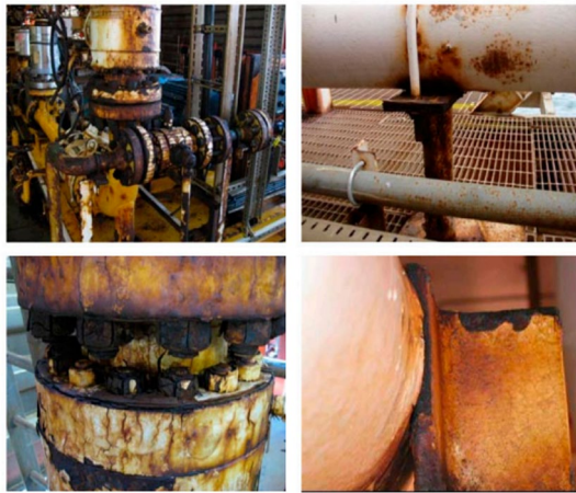
Fig. 3 Corrosion effect on bolt, flange and pipes [17]
